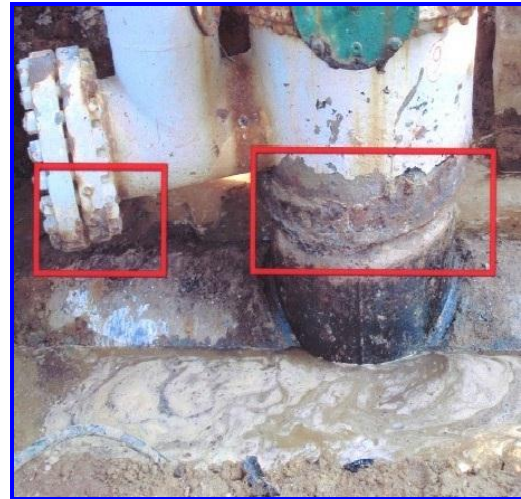
Area to be repaired
