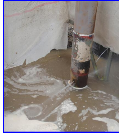
Area to be repaired with 3 pinhole leaks present
