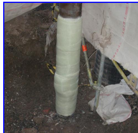
12 layers of Clock Spring Contour applied, the leak has been completely stopped
