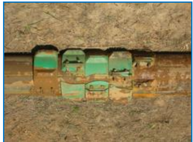
Spacers from old pipe, failed to stay in place when pipe removed – with corrosion
